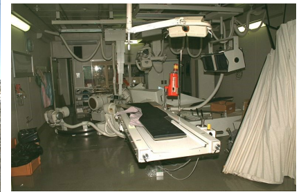
Figure 15: Non-structural Damage, Kobe Earthquake 1995
