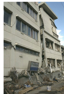
Figure 14: Structural damage, Kobe Earthquake 1995
