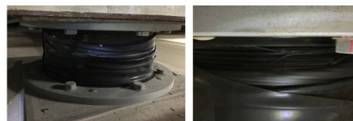
Figure 21: No damage of base isolation rubbers Aso Medical Center Source: Nikken Sekkei Archits. & Engrs
