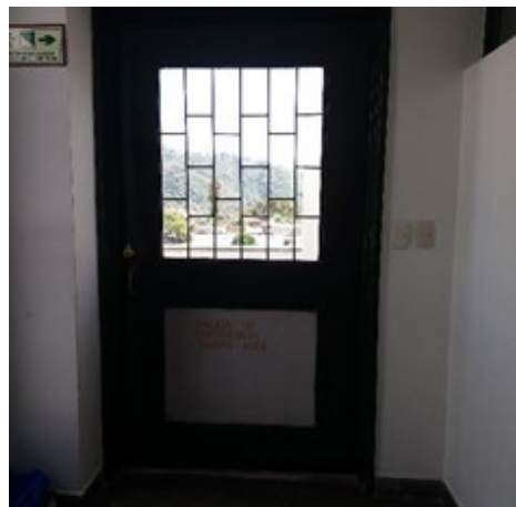
Figure 10: Blocked emergency exit
