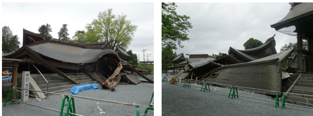
Figure 18: Aso shrine was completely crushed Source: Nikken Sekkei Archits. & Engrs
