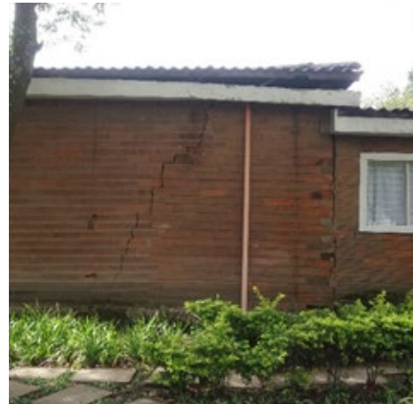
Figure 9: Dirt floor/lacking structural foundation
